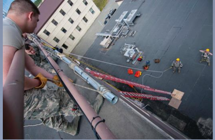
Members of the 176th Communications Flight prepare to mount an antenna on top of a building on JBER, Alaska May 26. (U.S. Air National Guard photo by Staff Sgt. Edward Eagerton)
