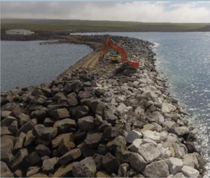
St. George Island Seawall. Repairs to the seawall began this summer and will conclude in 2017. Photo courtesy Brice Construction.
